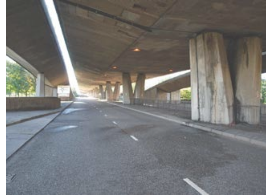
View looking north underneath the elevated Gateshead Highway towards the five bridges roundabout
